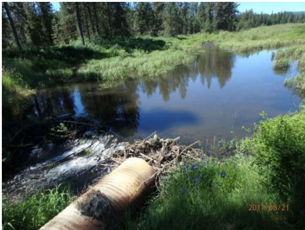
Figure B-40. Beaver dam and failed culvert at the bottom of Stranger 7 reach. This photo is representative of low gradient stream meandering through densely vegetated wetland. Numerous juvenile salmonids were observed on the margins of the channel here.
