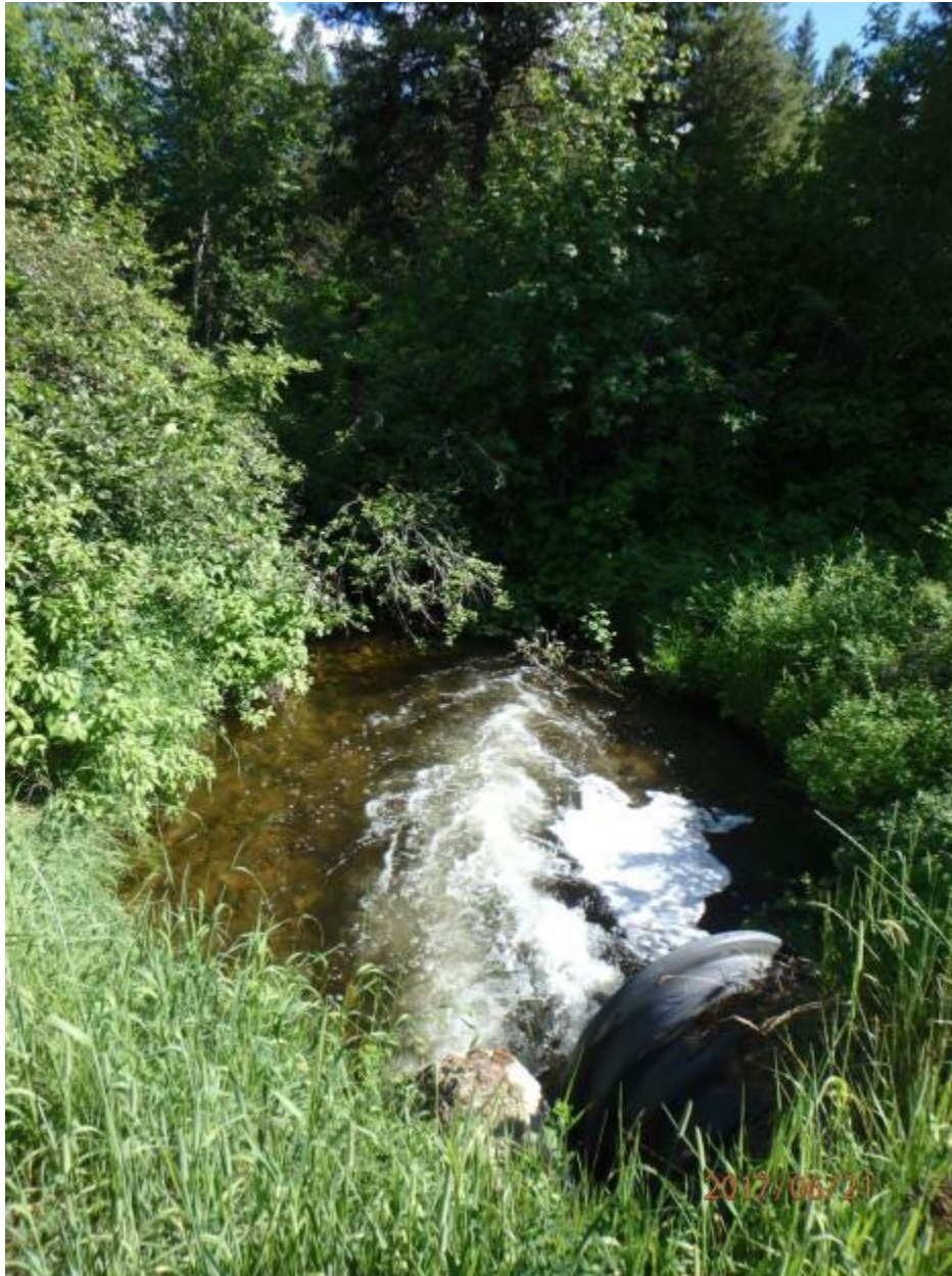
Figure B-31. Culverts at the top of NF Hall 1B reach. These culverts flow under a farm lane that does not appear to be necessary. Removal of these culverts or modification of the outlet with a boulder step configuration could be a relatively inexpensive and easy project.
