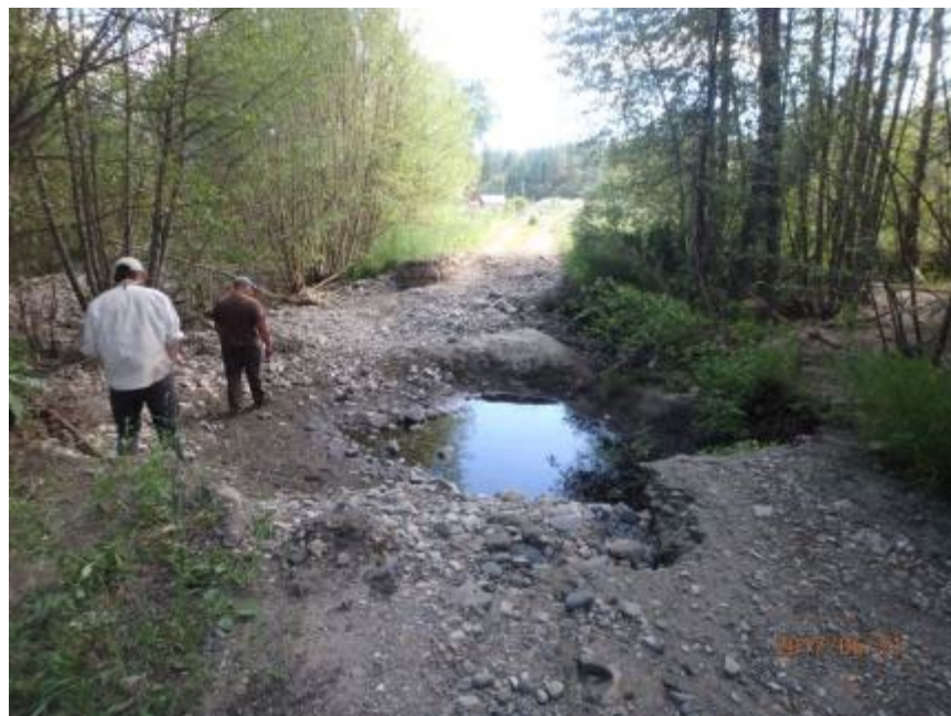
Figure B-62. Evidence of floodplain activation during April 2017 flood events. The road washed out here as the creek engaged a historic channel and sediment was delivered to the floodplain for several hundred meters downstream.
