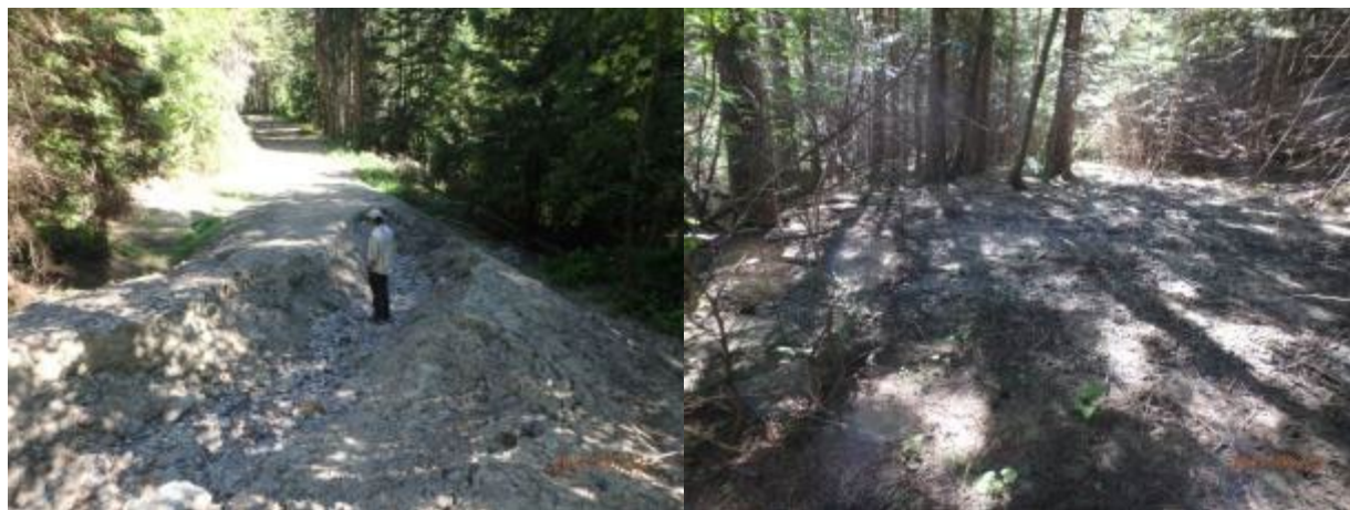
Figure B-53. Roadbed erosion caused during April 2017 storm (left panel). Right panel shows road sediments delivered across the forested riparian zone directly to Barnaby Creek.
