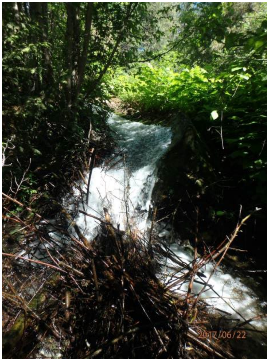
Figure B-11. Concrete overflow chute on the Cedar Creek dam. Overflow water drains from the pond surface and falls approximately 4 meters with a 1 m impassable drop to the stream bed at the bottom of the chute.
